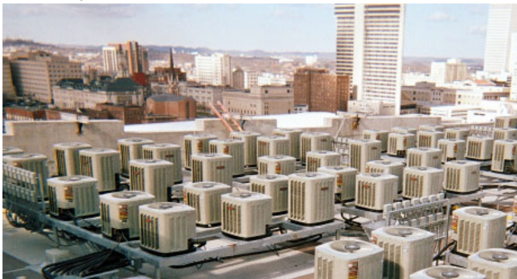
Photo for illustration purposes - area between units open for air to draw from top, bottom, and sides.
