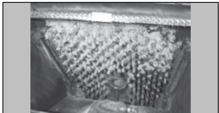
Figure 21.2 - Example of a dirty heat exchanger
