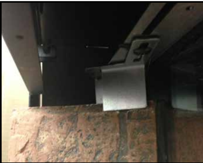
Figure 11.27 Side Refractory Brackets
