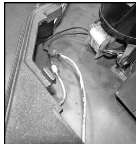
Figure 28: Note wire position.
