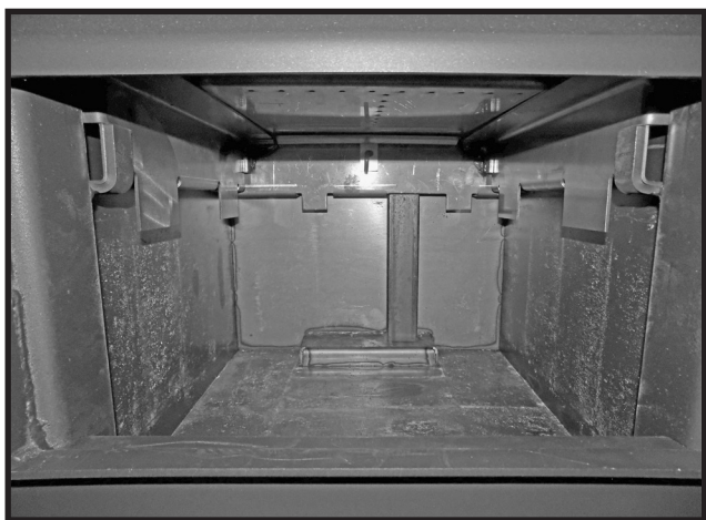
Figure 25: Chambre de combustion vide.
