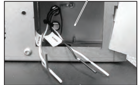
Figure 25: Junction box wiring
